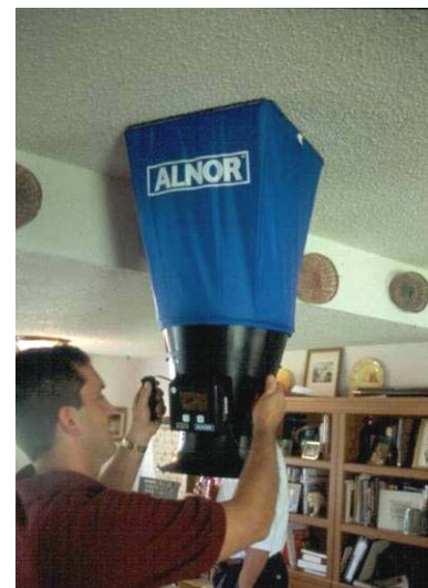
Figure 3. Testing for supply airflow balancing
